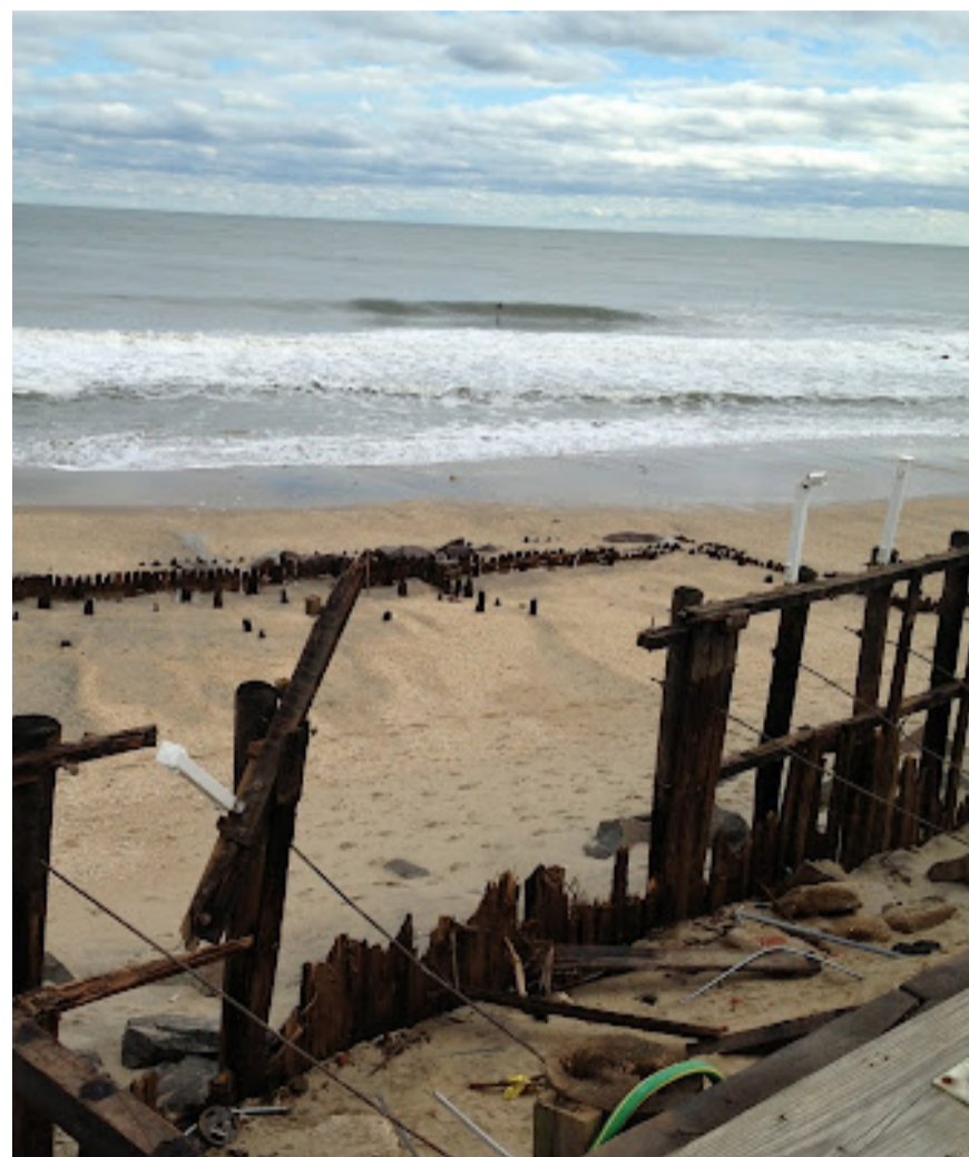
Remains of Harbour Mansion bulkhead days after Sandy
